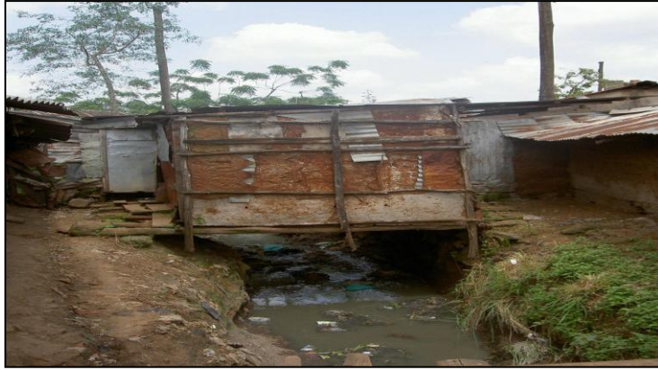
Fig-6: A photograph showing a pit latrine constructed across a river within the slum
